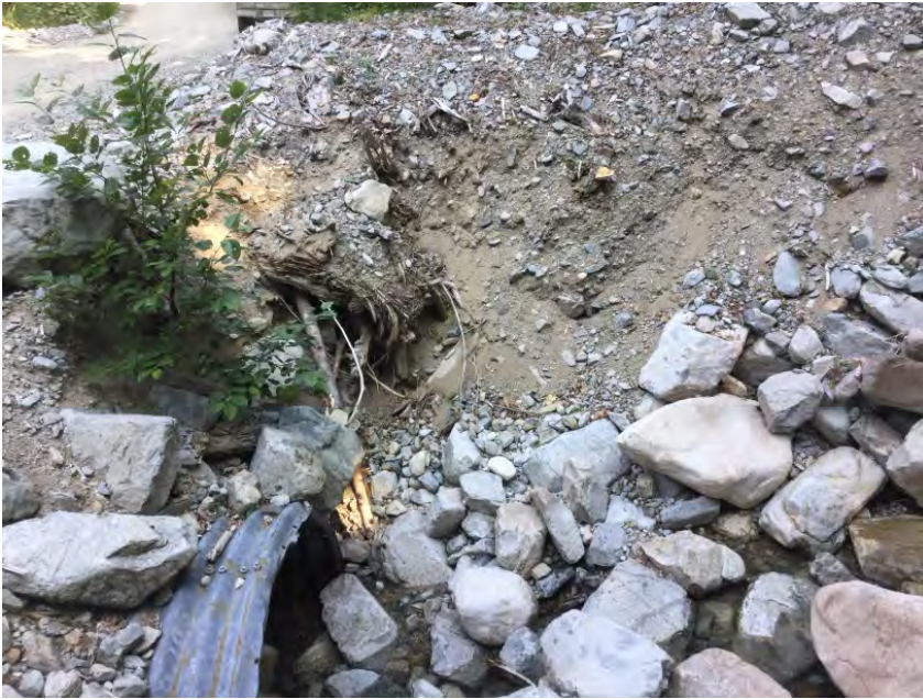
Organics and lack of riprap at inlet
