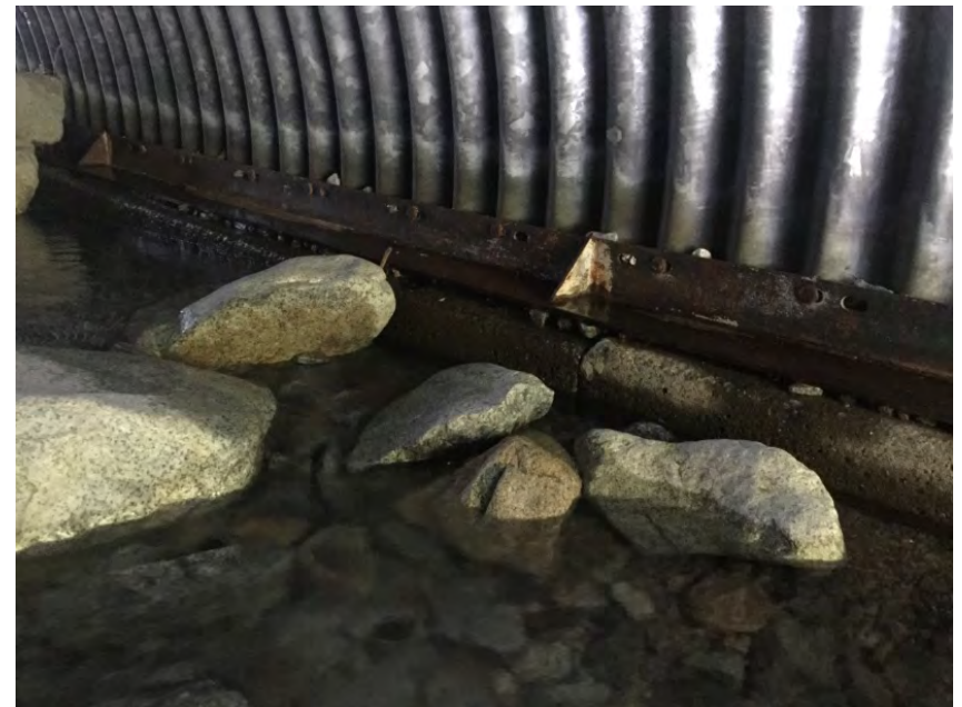
Consistent bearing on both footings, right bank settlement of left footing noted
